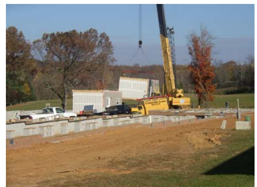
Clearance for the crane is a must. All obstacles must be considered.
