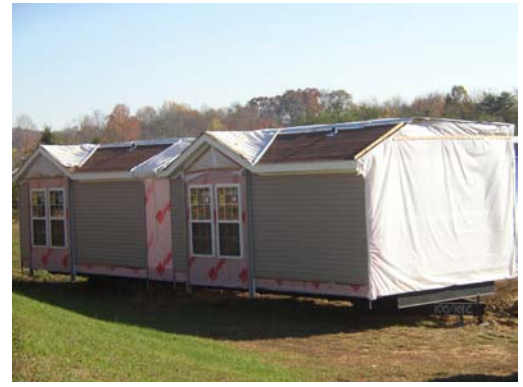
Units arrive onsite sealed against exposure and elements.
