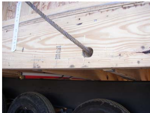
Crane rigging is installed on the units for movement to the foundation.
