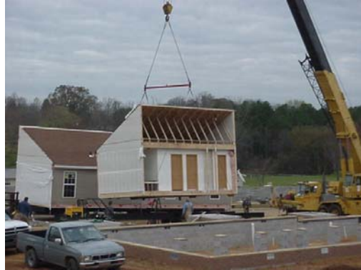
The roof is raised and second floor units are put in place on top of first units.
