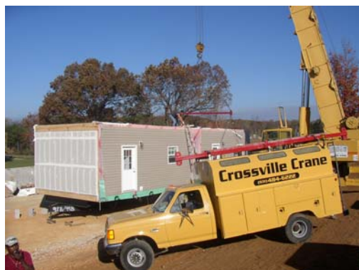
Rigging must be custom designed to each unit due to size differences.
